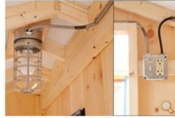
Electricity package with caged light, receptacle, switch and junction box outside for wiring
